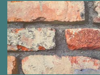
BRICK PLASTER CRUMBLE
